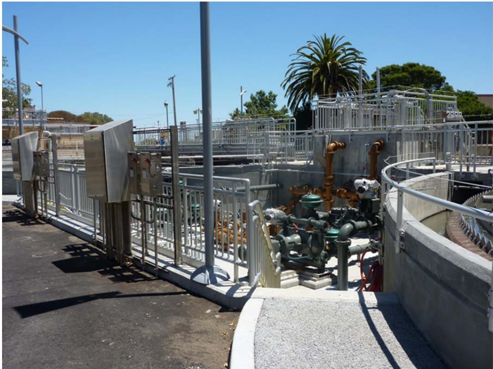
Treatment plant facilities
