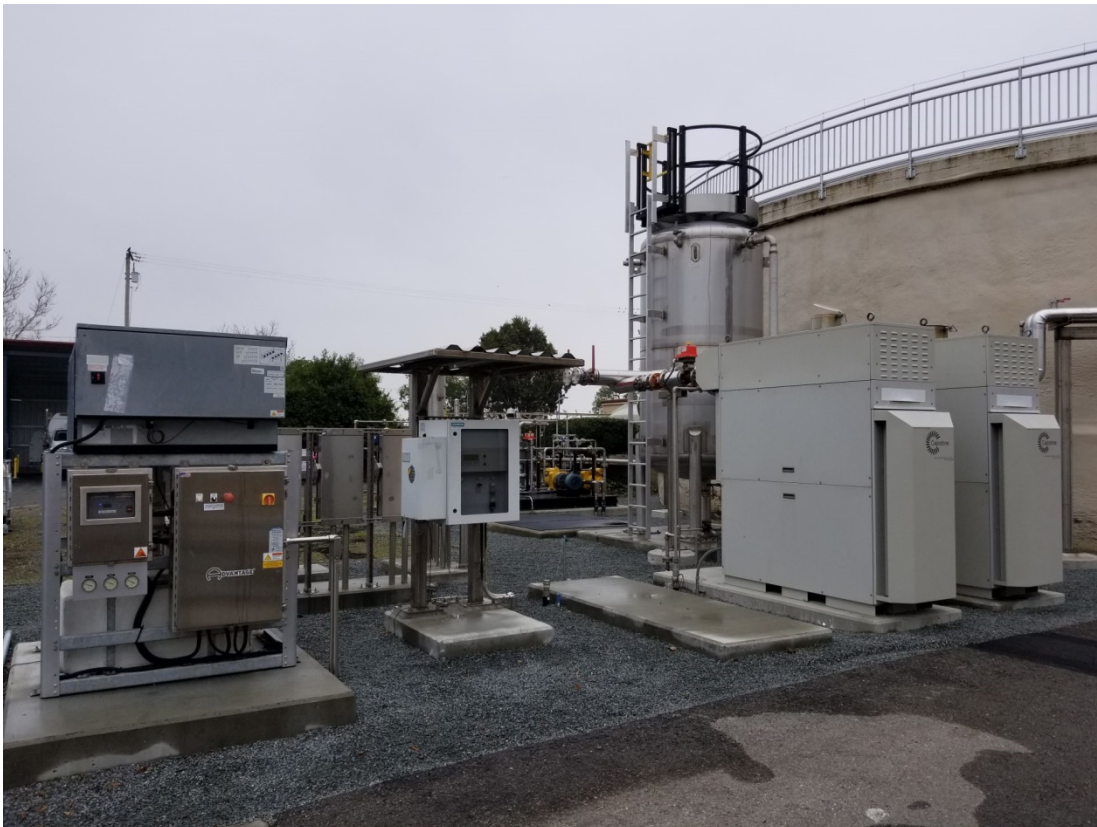
Biogas Recovery System Microturbines
