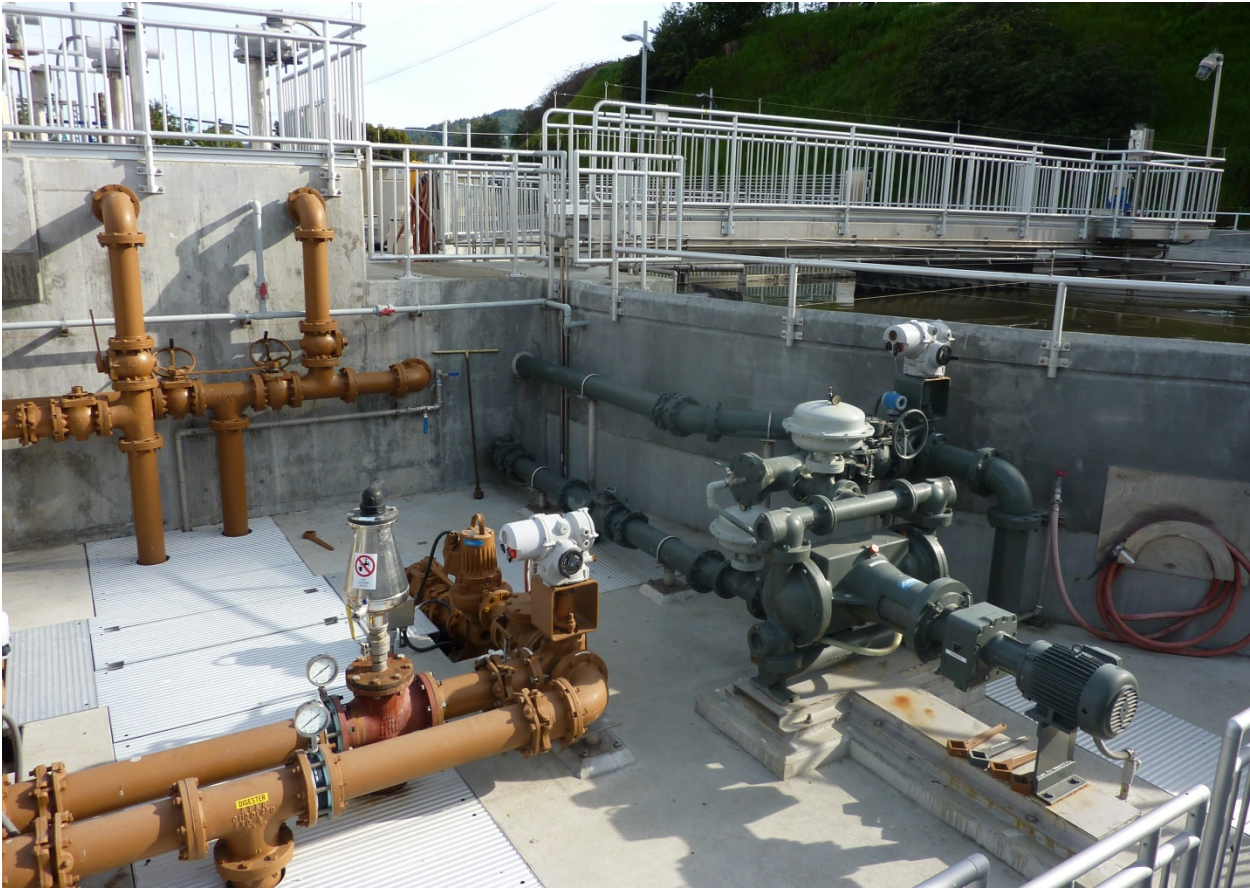
Primary clarifier sludge pump facilities
