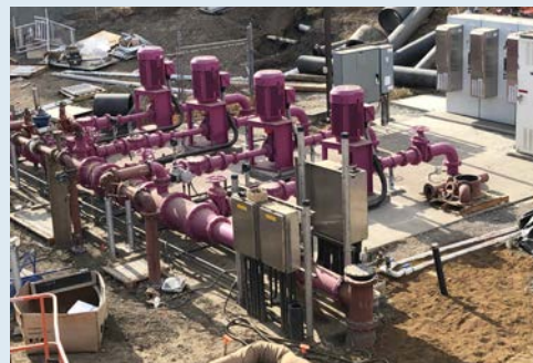
New Recycled Water Distribution Pump Station
