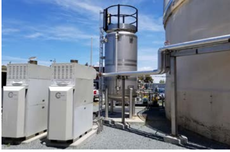
Methane Gas Powered Microturbines
