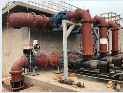
New Internal Recycle Pump Station
