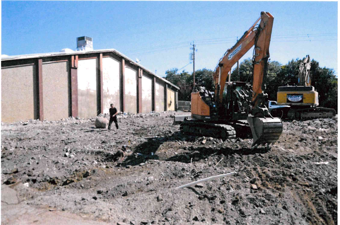
A crew clears debris after demolishing part of the Marinwood Plaza Shopping Center in 2022. An affordable housing project sought at the site could get county approval within 120 days. PHOTOS BY ALAN DEP — MARIN INDEPENDENT JOURNAL
