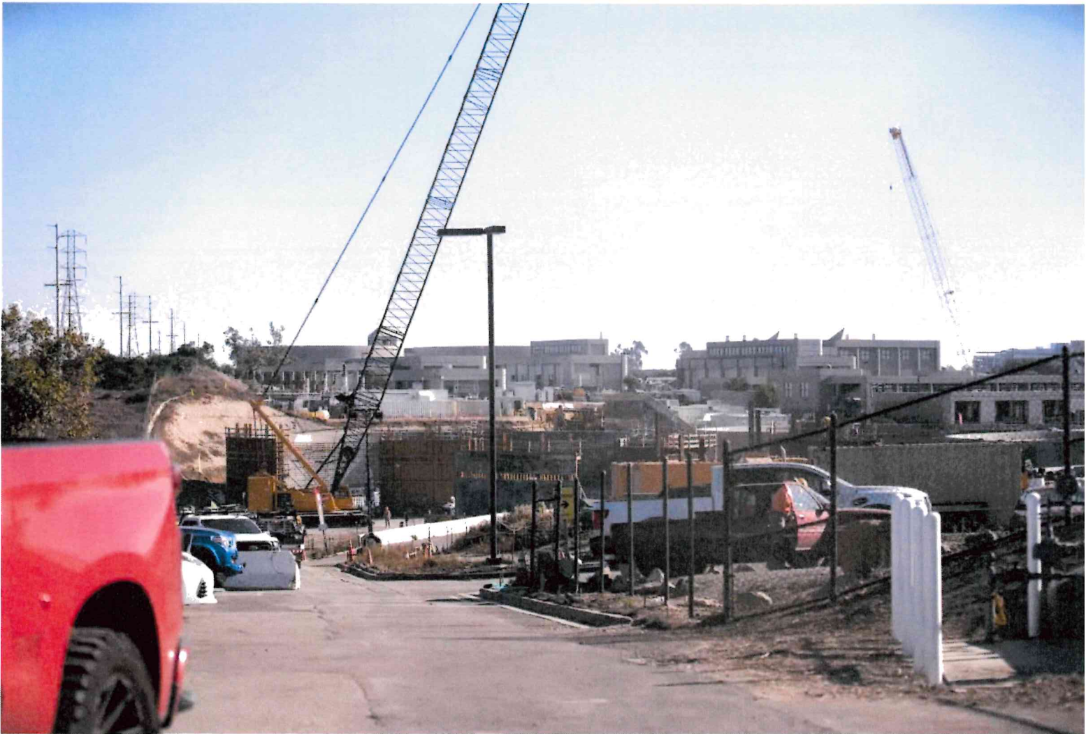
Pure Water construction at a recycling facility in San Diego. (Ana Ramirez/The San Diego Union-Tribune)
