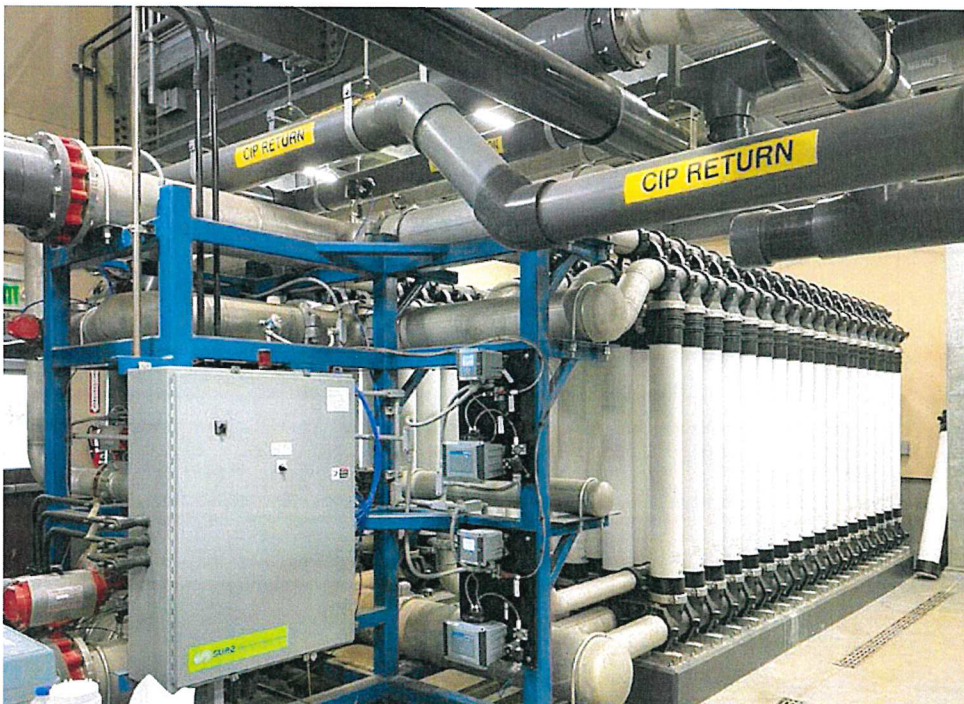
Recycled water membrane filter system
