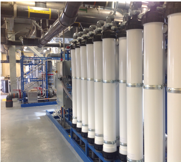
Interior of District's Recycled Water Plant
