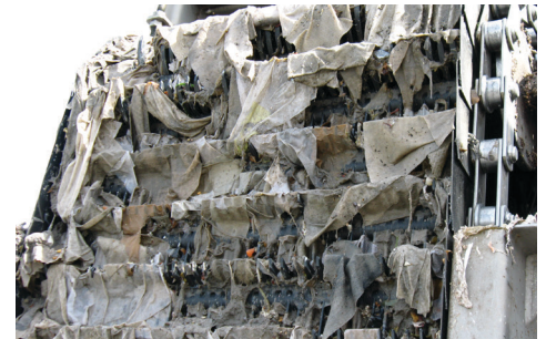
Screens installed in 2006 were part of an over-$4 million project to help protect the treatment plant from personal wipes.
