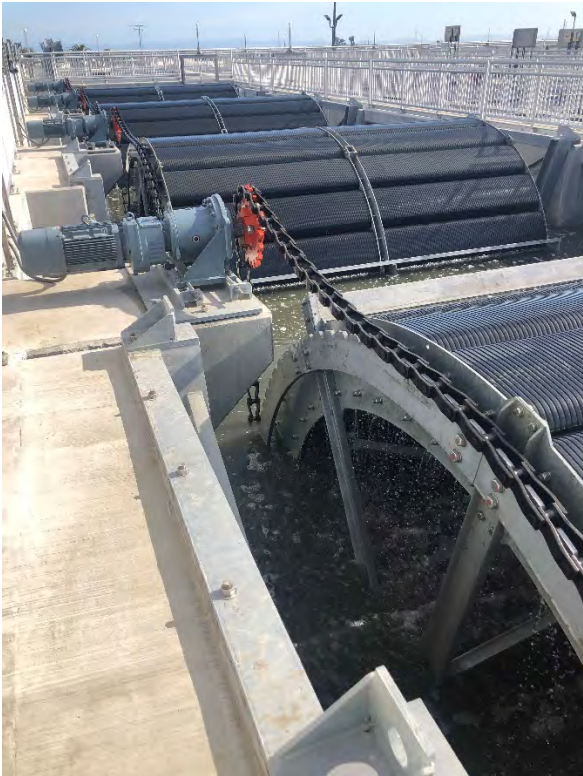
Commissioning of the BioWheels Aeration Tanks in March 2021
