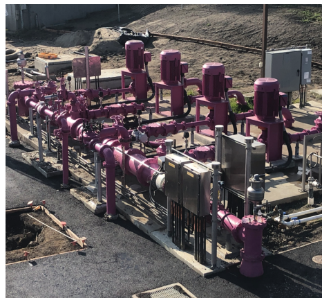
New Recycled Water Distribution Pump Station
