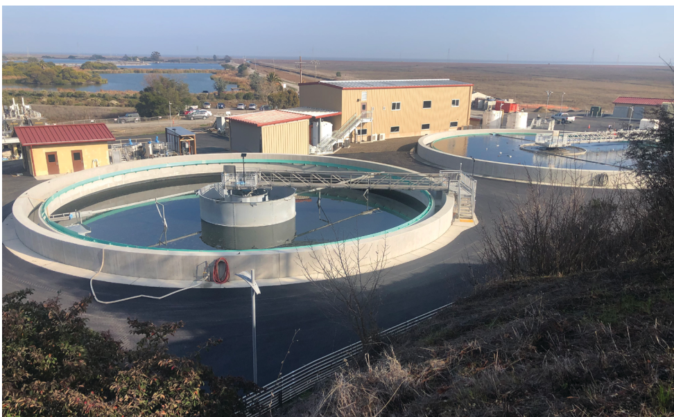
New wastewater clarifiers are part of the recently completed Secondary Treatment Plant Upgrade and Recycled Water Expansion Project.
