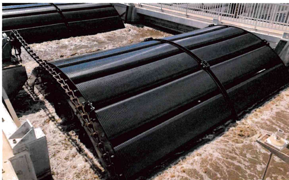
Top: One of the two new secondary clarifiers. Bottom: New aeration basin with bio-wheels.
