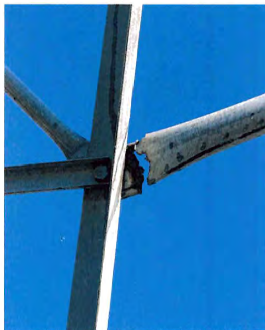
Figure 2. Separation at Center Pivot No. 1 Mechanism.
