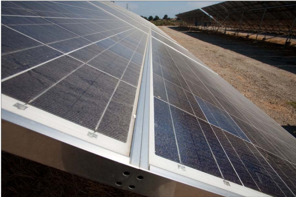
Photovoltaic Panels Generate Power for the Treatment Plant
