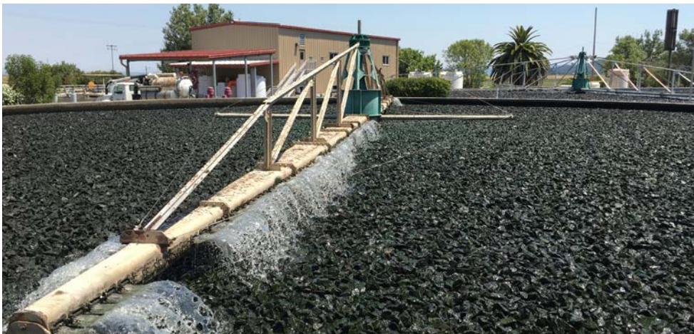
LGVSD's secondary biological process equipment, including trickling filter shown above, are over 60 years old and at the end of their useful life.
