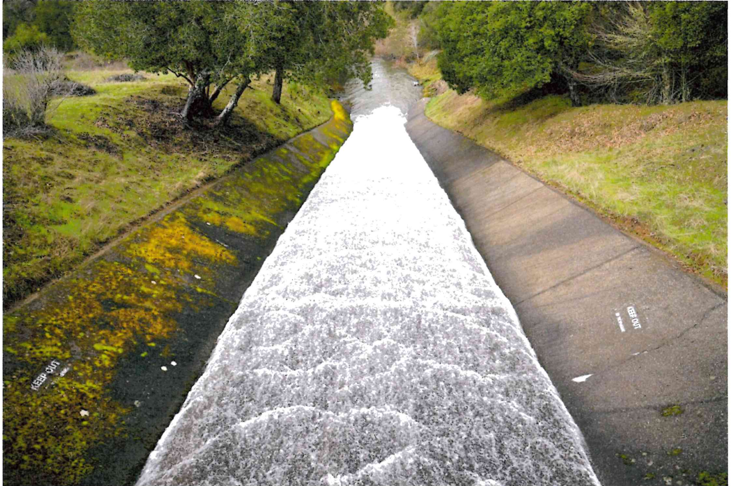
Runoff flows down the Bon Tempe spillway in Fairfax on Wednesday. A series of storms brought the Marin Municipal Water District reservoirs to 100% capacity this week. PHOTOS BY SHERRY LAVARS — MARIN INDEPENDENT JOURNAL
