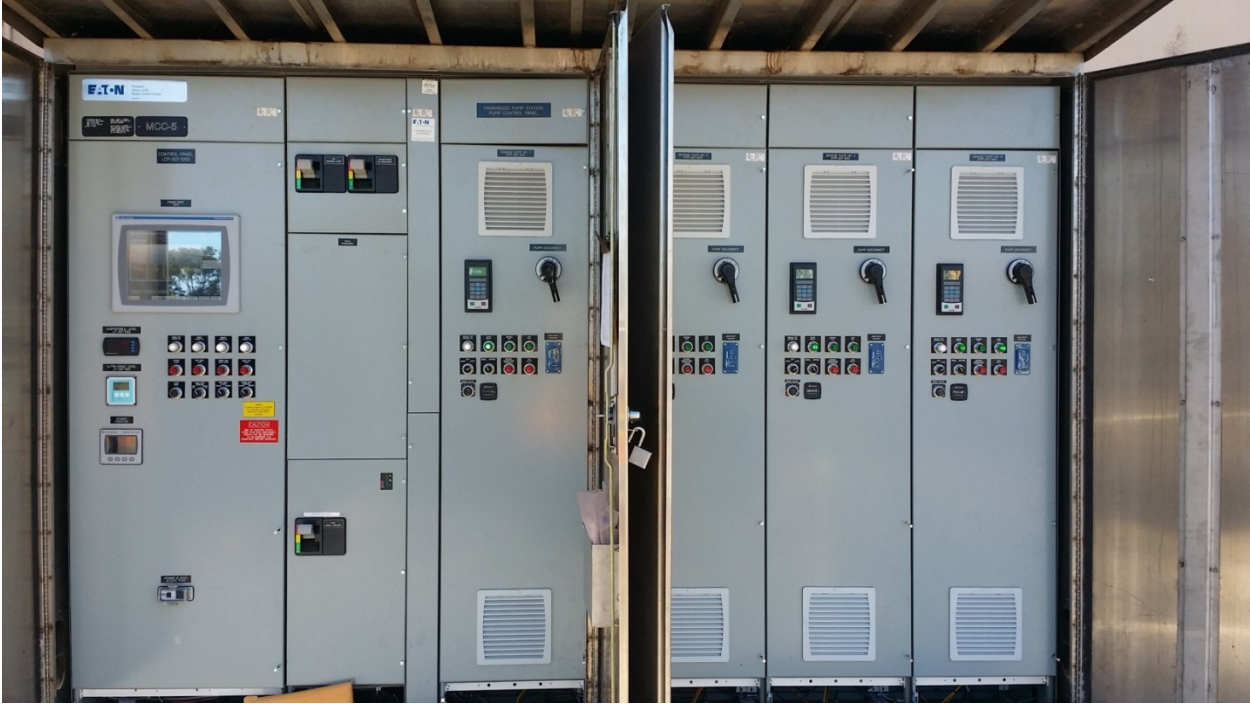
Marinwood Pump Station motor control center
