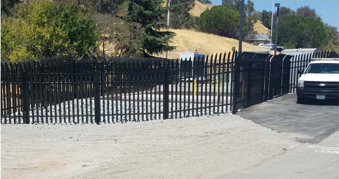
Compressed natural gas fueling station for the new vehicle
