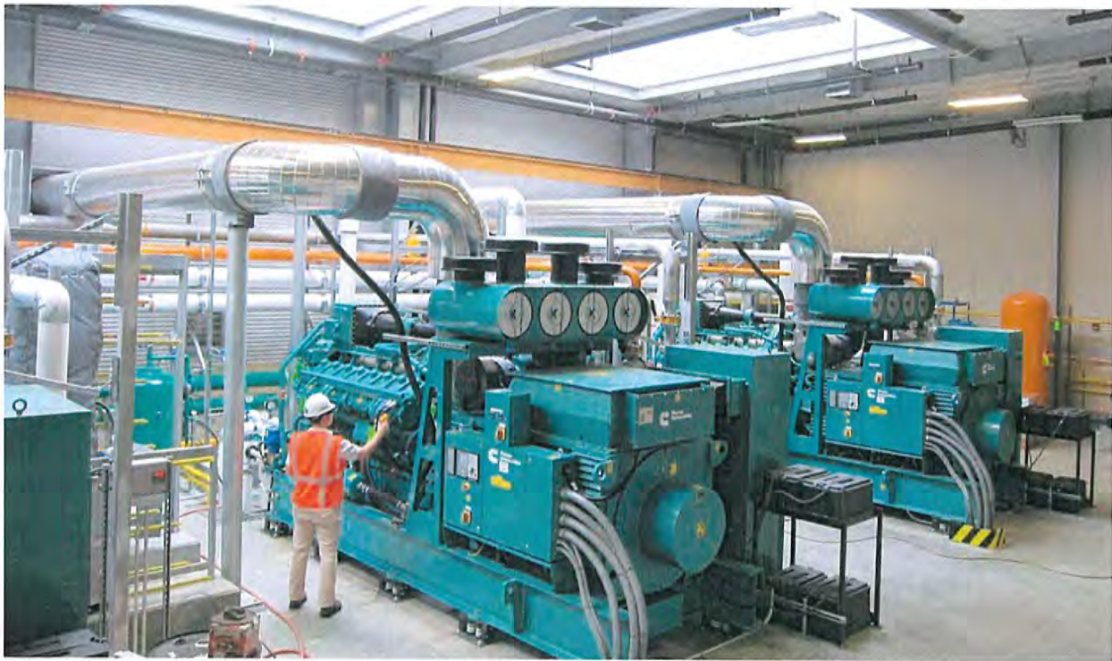
Figure 4. Santa Rosa's CHP facility has four 1100-kW engines
