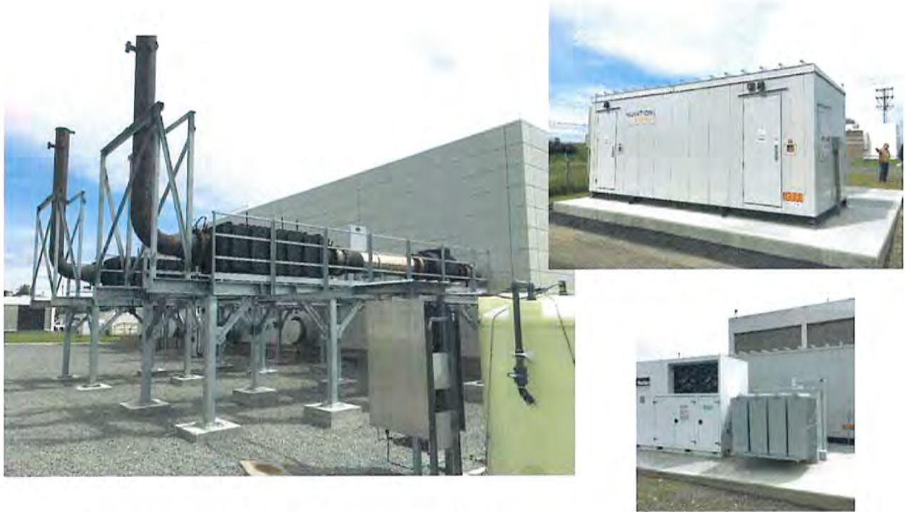
Figure 7. Components of the City of Santa Rosa's Microgrid Demonstration facility – microgrid controller, battery energy storage, and selective catalytic reduction emissions control for natural-gas engine operation
