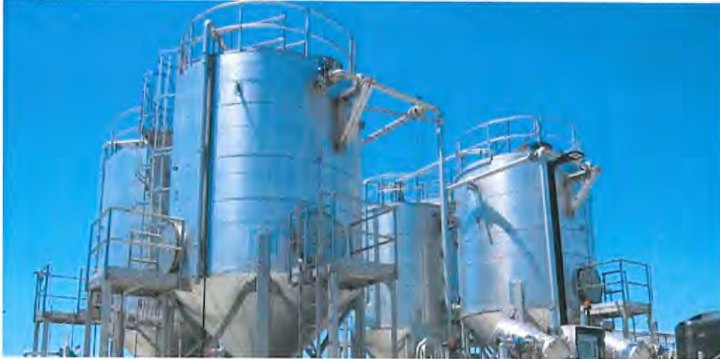
Figure 6. Santa Rosa’s HSW Receiving Tanks
