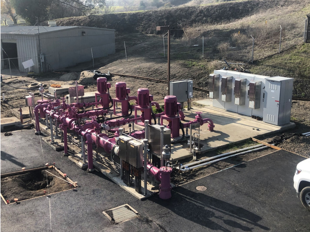
Distribution pump facilities
