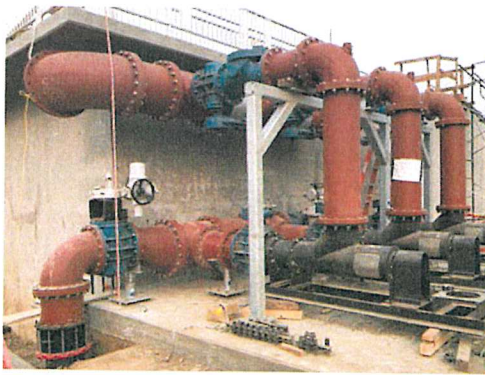
New Internal Recycle Pump Station
