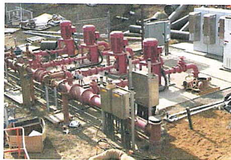
New Recycled Water Distribution Pump Station
