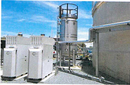
Methane Gas Powered Microturbines
