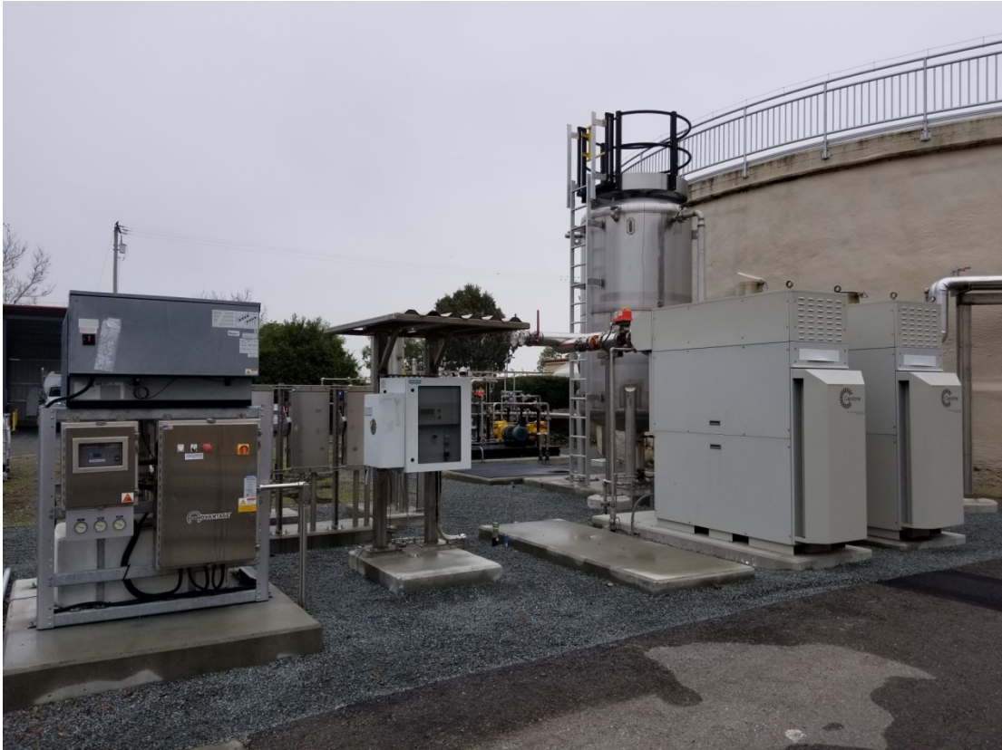
Biogas Recovery System Microturbines
