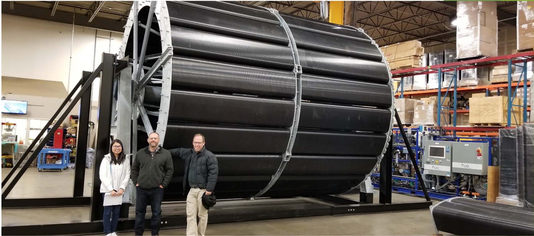
Treatment plant upgrades - 1 of 16 BioWheels
