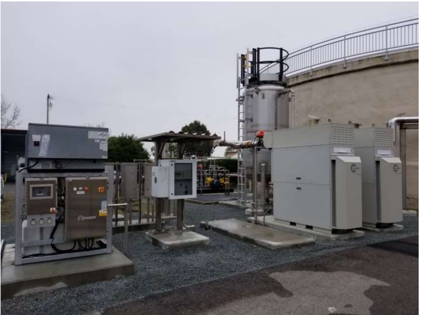
BERS Microturbines in Operation
