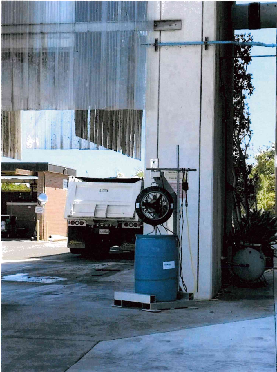
One of six odor-mitigating fans at the Vallejo wastewater treatment plant. Vallejo Flood and Wasterwater District
